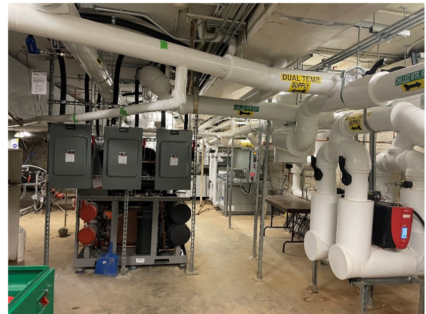
Figure 6. City Hall Mechanical Room
